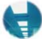
LV energy cables
